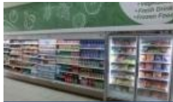
Energy saving at convenience stores, Panasonic, Indonesia
