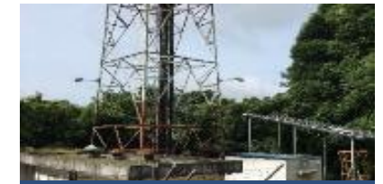
Energy-saving of mobile communications base transceiver stations, KDDI Corp. Indonesia
