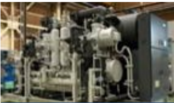
High-efficiency refrigerator, Mayekawa MFG, Indonesia
