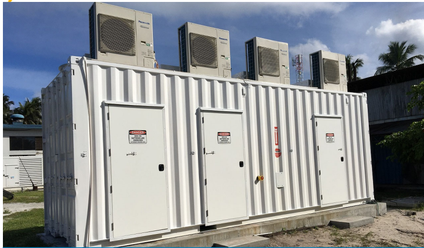
BESS under operation
