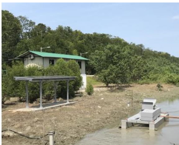
Float-type Micro Hydropower Facility
