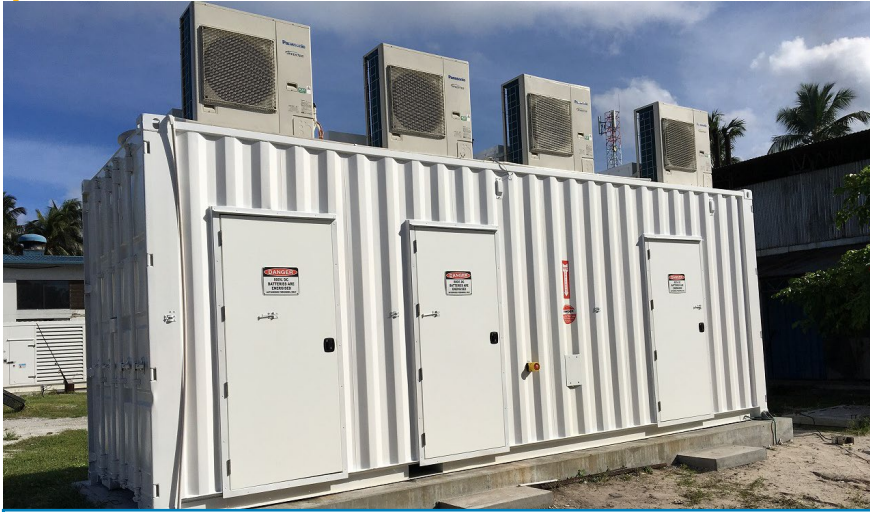
BESS under operation
