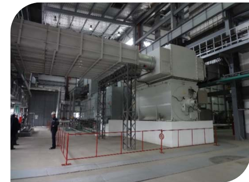
Gas turbine room
