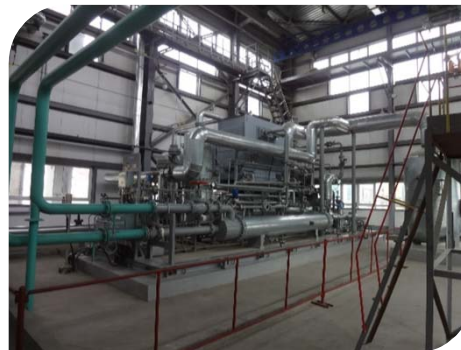
Heat exchanger room
