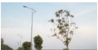
LED street lighting system with wireless network control, MinebeaMitsumi, Cambodia
