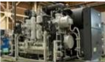
High-efficiency refrigerator, Mayekawa MFG, Indonesia
